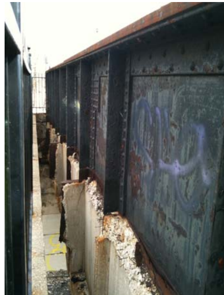
11 th Street Space between Bridge and Sidewalk
